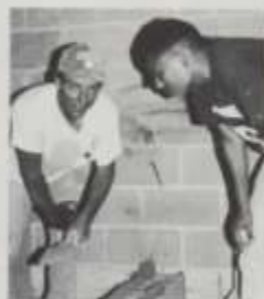
Chris Jones watched Ray Johnson as he constructed booths for the ag department. Johnson showed the students the art of masonry after they missed the marts for him.
